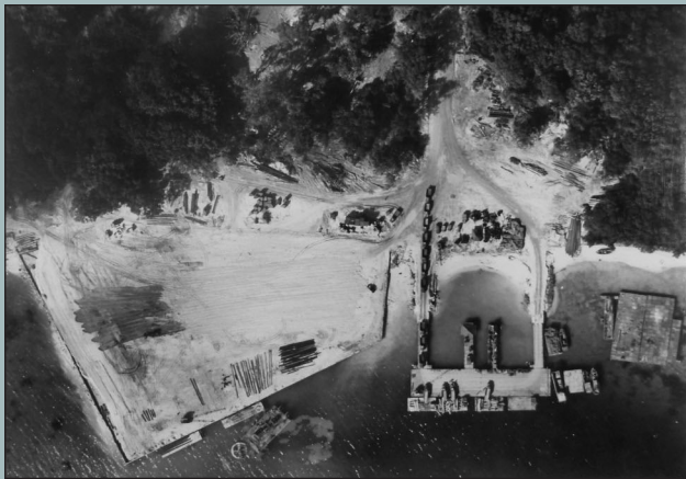
The slipways and dockside infrastructure under construction at the supply depot. Photo – US Archives.
