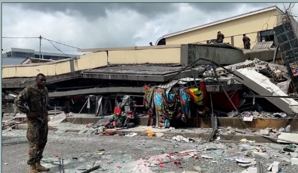
The Billabong building in downtown Port Vila became the centre of the relief effort with many people trapped alive under the building. Photo – Various sources.
