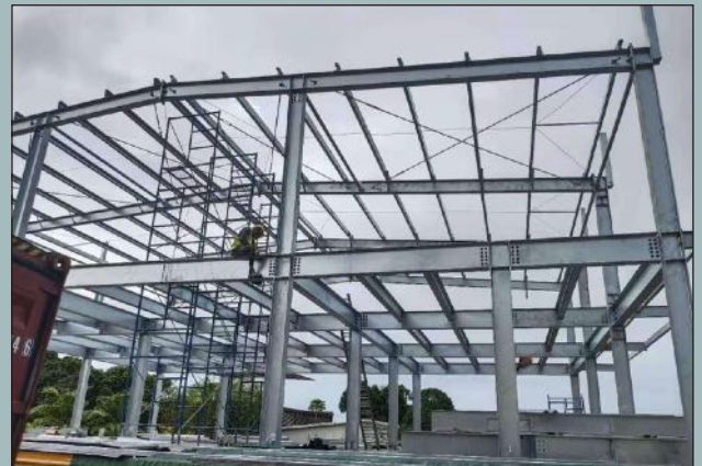
A steel frame office building being built in Vanuatu. Modern construction techniques will help lessen the effects of natural disasters. Photo – Director Group DFX.
