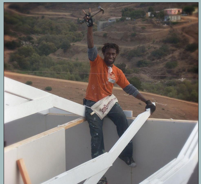
Lemy hard at work building a home in Mexico some years ago.
