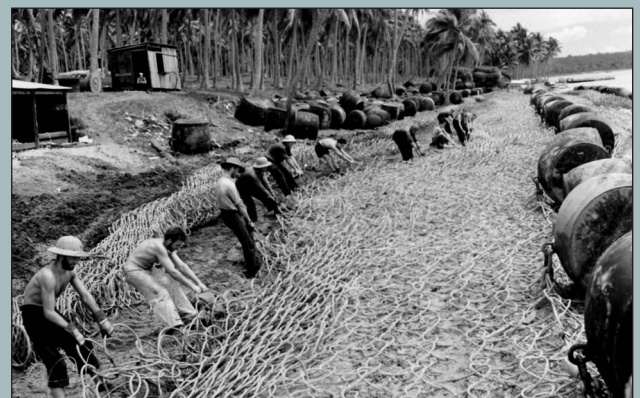
US Navy Seabees 'weave' anti-submarine netting to be positioned across the Segond Channel. Photo – US Archives.
