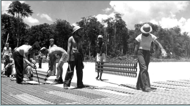
Bomber #2 airfield during construction. Marston matting is being laid by Navy Seabees. Photo US Archives.
