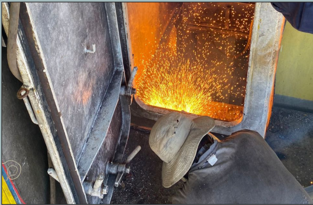
The cutting crew torch the door and its frame from the ship.
