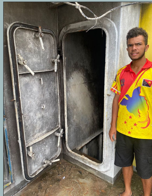
Bradley's son Jaden stands with the door prior to it being cut out of the ship.
