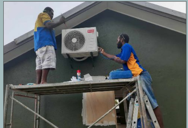
The air conditioning unit gets affixed to the rear of the museum.
