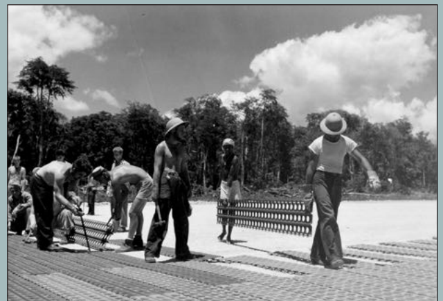
Construction of Bomber Airfield #2 by US Navy Seabees Assisted by local Ni-Vanuatu workers.
