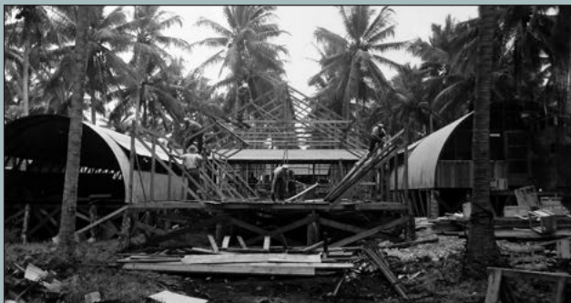
Construction of three Quonset hits joined together to make one large mess building on Espiritu Santo in 1942.
