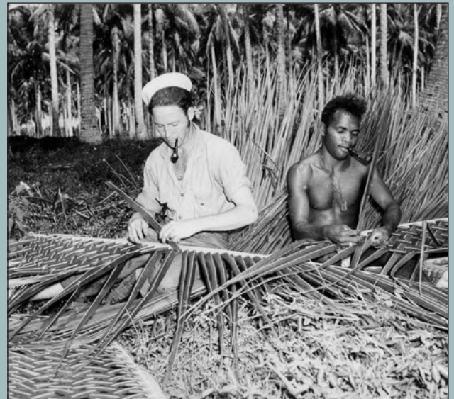
A local Ni-Vanuatu teaches a US Navy Seabee the fine art of traditional weaving palm leaves for roof and wall sections.
